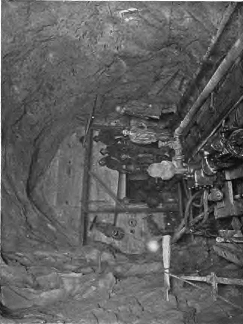
PLATE 189. —Contract 90. Concrete Bulkhead at East Shaft Hudson Siphon. Its purpose was to safeguard shaft in case of sudden inflow of water while excavating heading. Designed to withstand head of 1100 feet. It was never necessary to close door.
